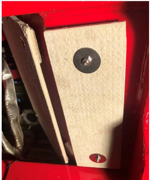
New HardiBacker cement board insulation panels in place (with proper spacers this time!)
