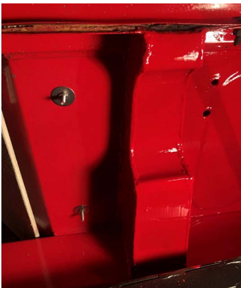
Unprotected section of flooring that contributes to "Healey Hot Foot". Stainless steel hardware and anti-seize compound should keep these fasteners from becoming a problem down the road.
